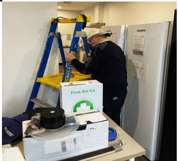
One of the volunteers (Fred Pither) giving the lunch room walls a fresh coat of paint.
